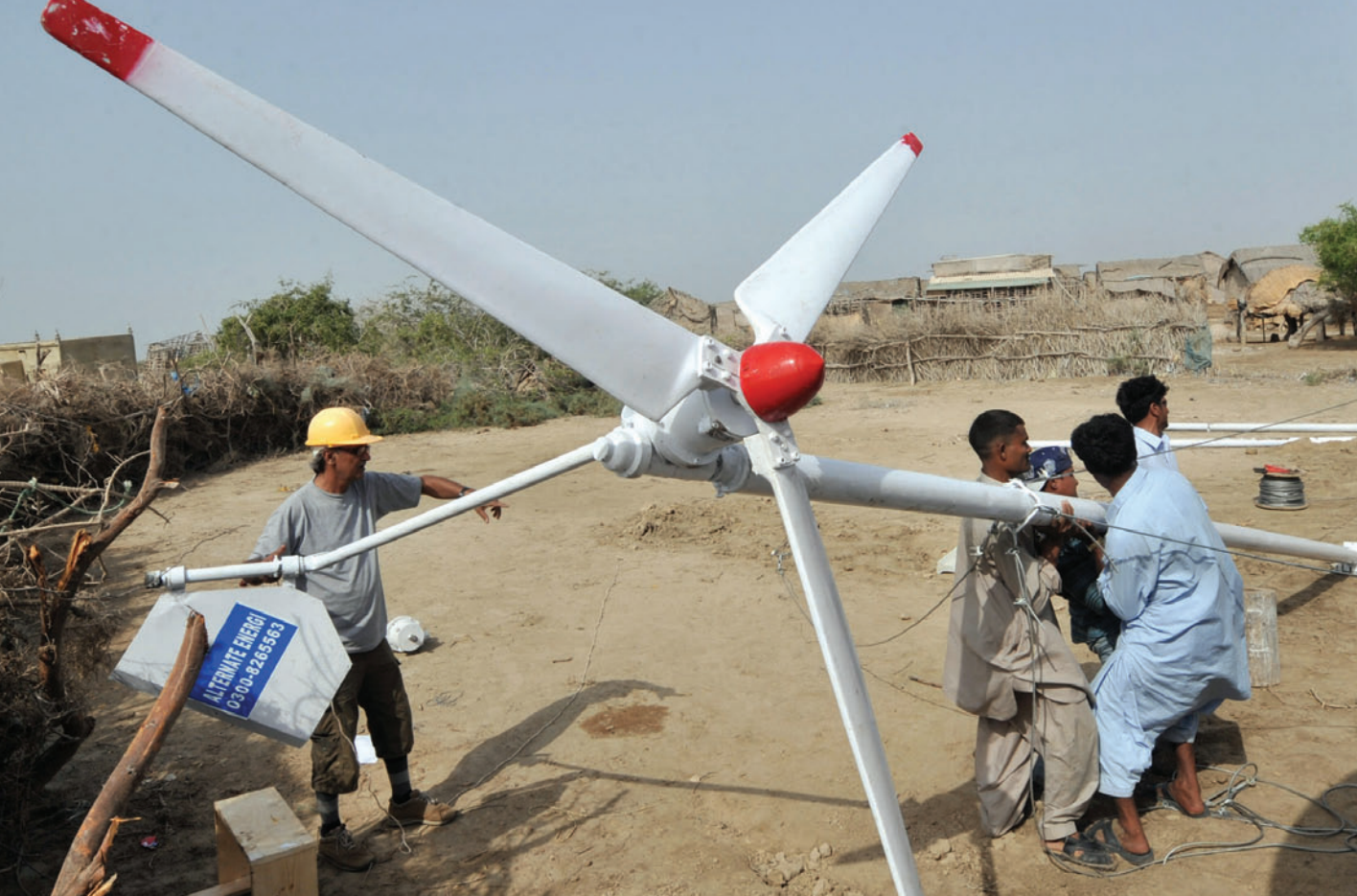
Pakistani technicians install a wind turbine on the subtropical island of Kharochhan, couched in the cyclone belt of the Arabian Sea. This tiny island is light years ahead of the country, powering homes and businesses with wind turbines, saving the ecosystem and improving residents' quality of life. | AFP Photo: Rizwan Tabassum
