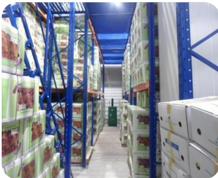
An example of an improved cold storage facility in Baluchistan funded by USDA and run under private ownership. Expanded cold storage has reduced losses of perishable produce, increased the shelf life of farmers' output, and expanded market reach. (USDA)
