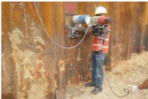
Collecting a concrete core sample of the containment structure to analyze the insulating value after Phase 1 treatment
