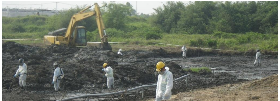
Excavating contaminated sediment in western portion of Sen Lake (Photo: CDM Smith)
