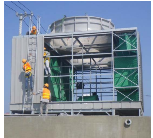
Liquid/vapor treatment system's cooling tower (Photo: CDM Smith)
