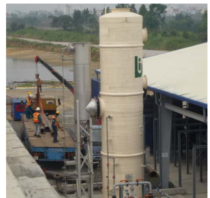
The liquid/vapor treatment system's quenching tower (Photo: CDM Smith)
