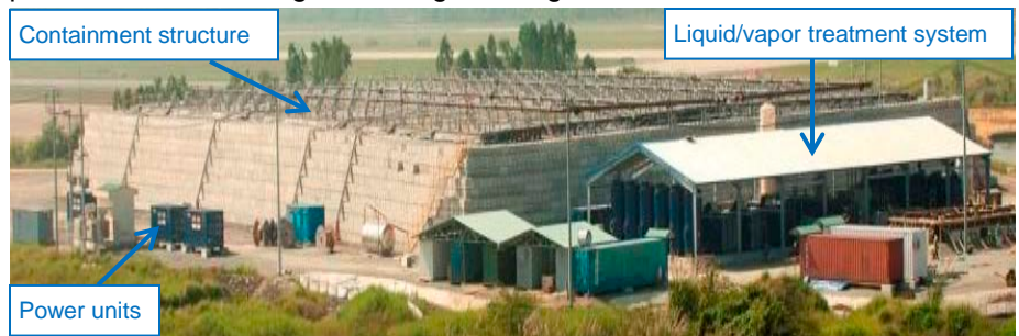
Containment structure and liquid/vapor treatment system (Photo: Tetra Tech)
