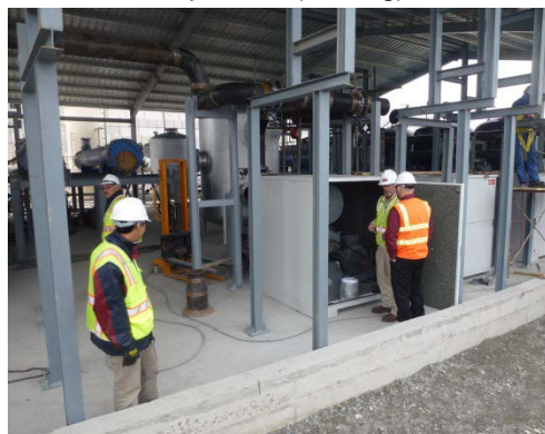
USAID contractors inspecting the liquid/vapor treatment system's blowers (Photo: CDM Smith)
